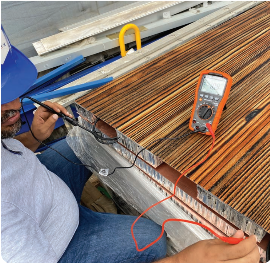
Testing Voc of Facade Solar Panels
