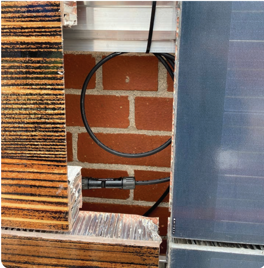
Panel to panel wiring hid behind the panels & run through conduit.
