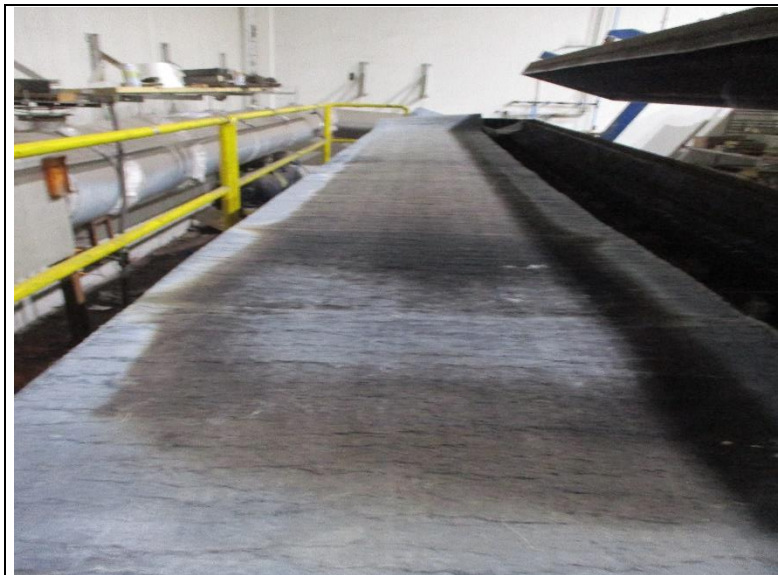
Photo No. 2 Post-Test
