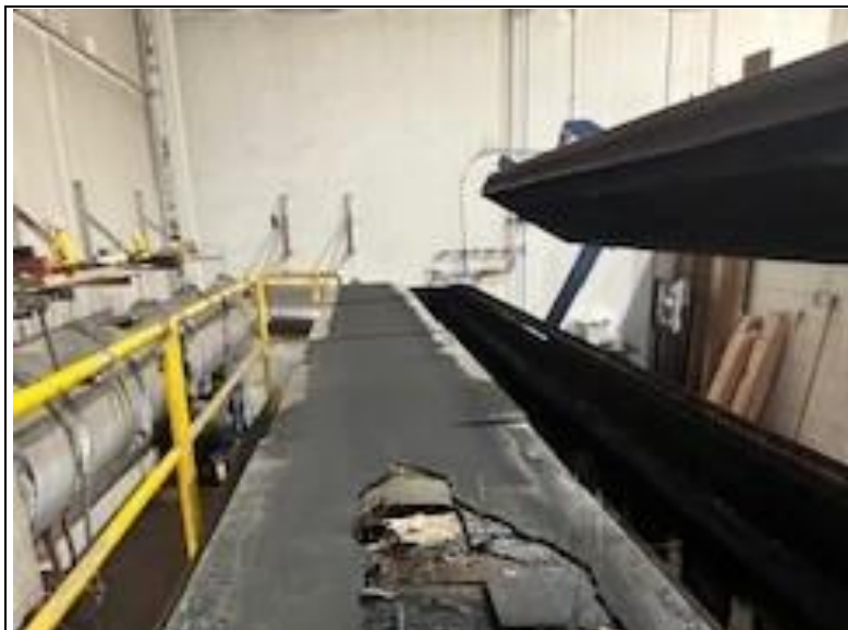
Photo No. 2 Post-Test
